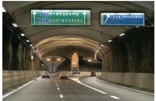
Long life illuminates Sweden's largest road tunnel construction, Södra Länken, even in cold temperatures.
